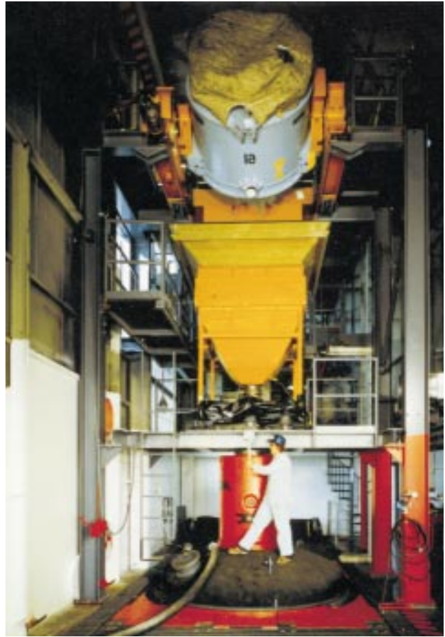
Figure 5-3: A propellant casting pit, with a motor case being cast below ground.
